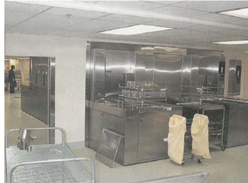
Two new washer/sterilizer machines were installed as part of this renovation project. This is a view of the clean side unloading area, looking through the door separating the clean side from the soiled side.
