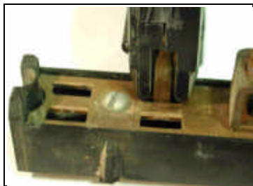
A. Copper buss bar with punched openings.
