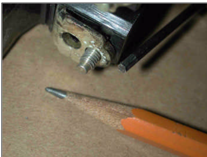
FIGURE 7 - ONE LOAD-SIDE CONTACT AND ITS 8-32 CLAMPING SCREW, ON THE FPE 100-AMP MAIN BREAKER OF FIG. 6. THE SCREW-HEAD TAKES A 3/32" ALLEN WRENCH, WHICH IS ONLY SLIGHTLY LARGER THAN THE LEAD OF THE #2 PENCIL.
